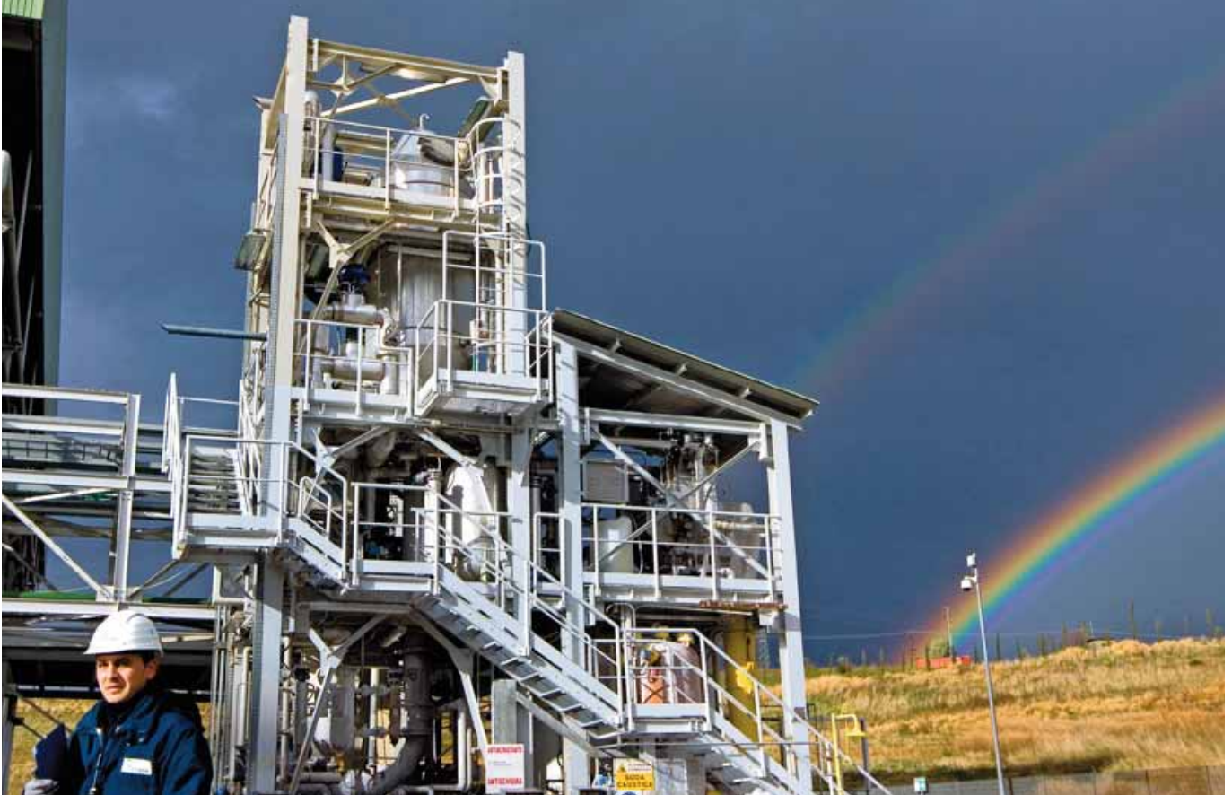
Combined-cycle gas turbine plant at Altomonte. All of EDF's generation facilities have been awarded environmental certification.
